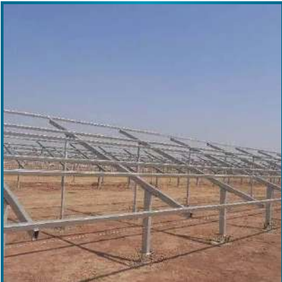
GI Solar Panel Mounting Structure
